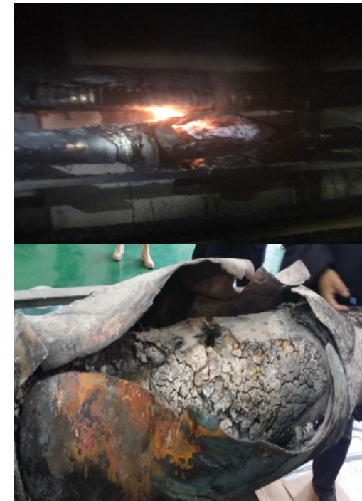
220kV Cable PMJ Breakdowns
